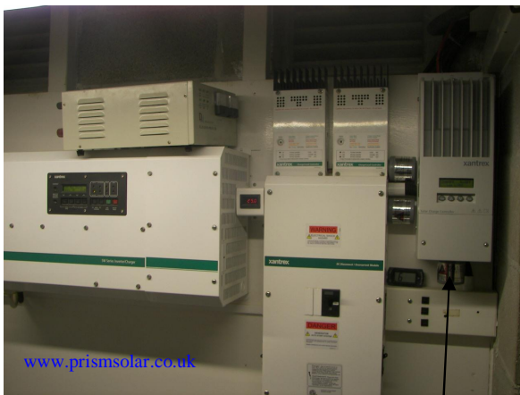
Here is the new XW60-MPPT sat to the right of the 2 x Xantrex C40 controllers. You can see that it is physically a lot larger the C40 range. The 3 Silver cans wired to the Charge controllers are Delta LA302DC lightning arrestors.
